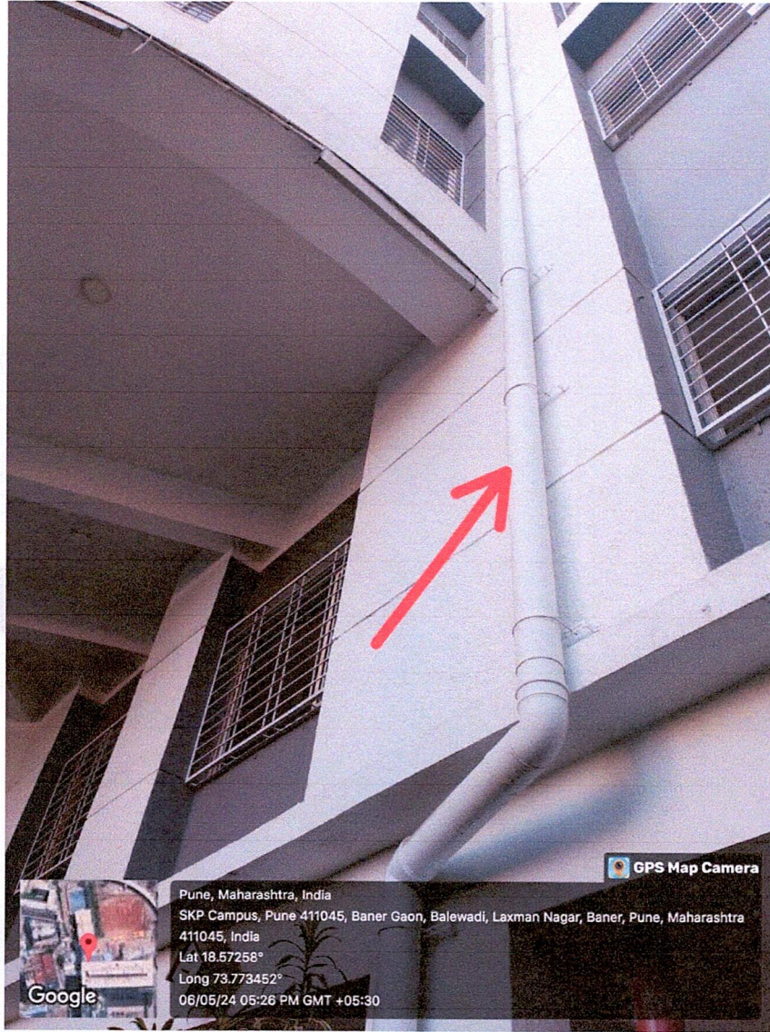
Pipeline of Rain Water Harvesting
